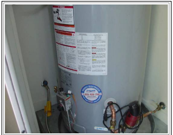
Hot water heater with recirculation pump
