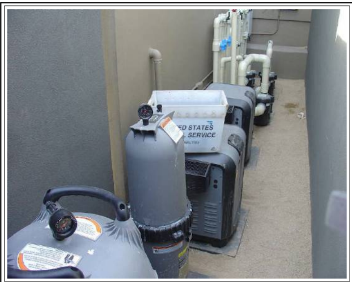
Pool filter equipment and pool heating system
