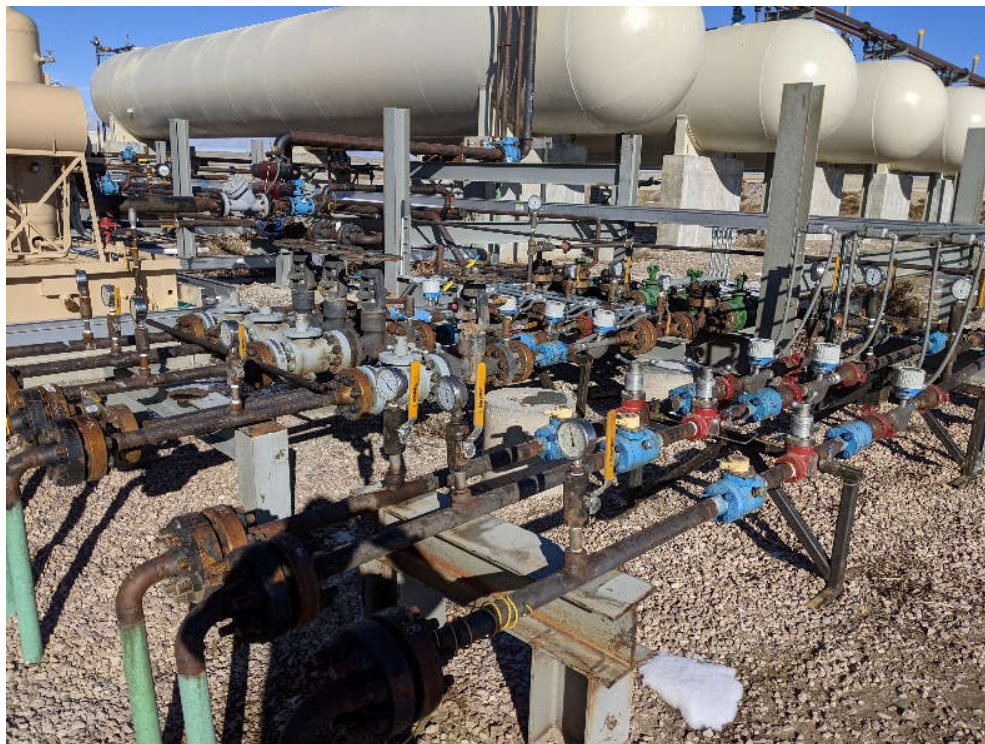
Figure A-7: The injection well manifold (working pressure 4,000 psi), coming off the discharge line of the second stage compressor
