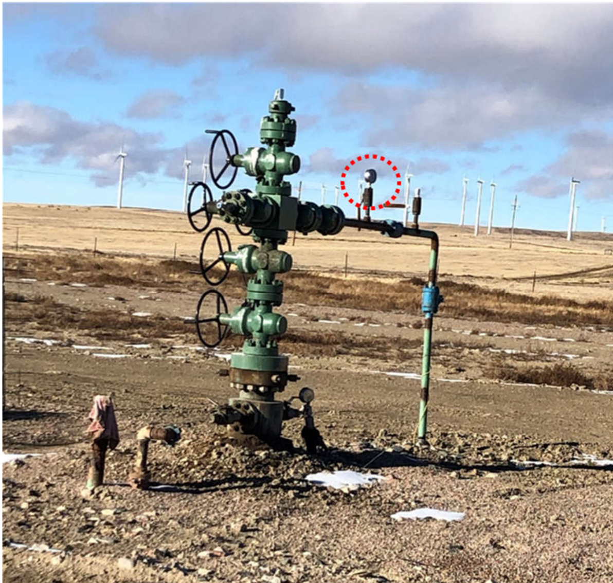
Figure A-8: A sample gas injection well, with the pressure gauge circled in red, chokes are down stream of the gauge
