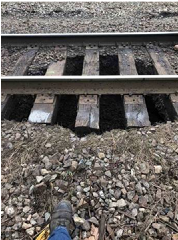
Figure 2 - Sinkhole formation at location of damaged sewer
