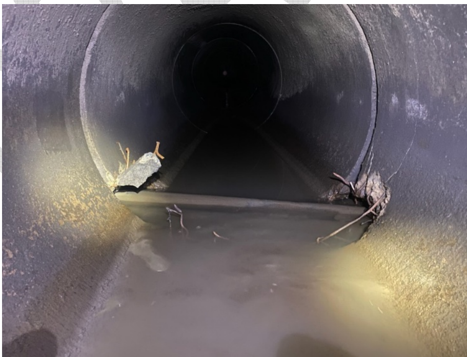
Figure 3 - View of damaged sewer & conduits installed
